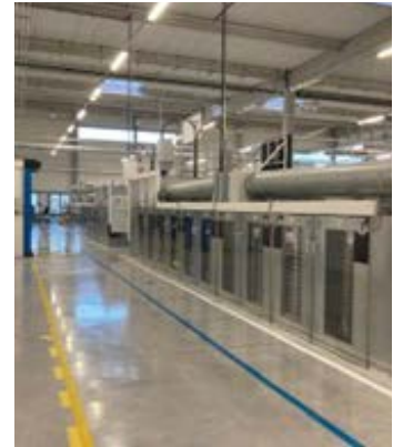
Conditioning tunnels in the Collégien plant
